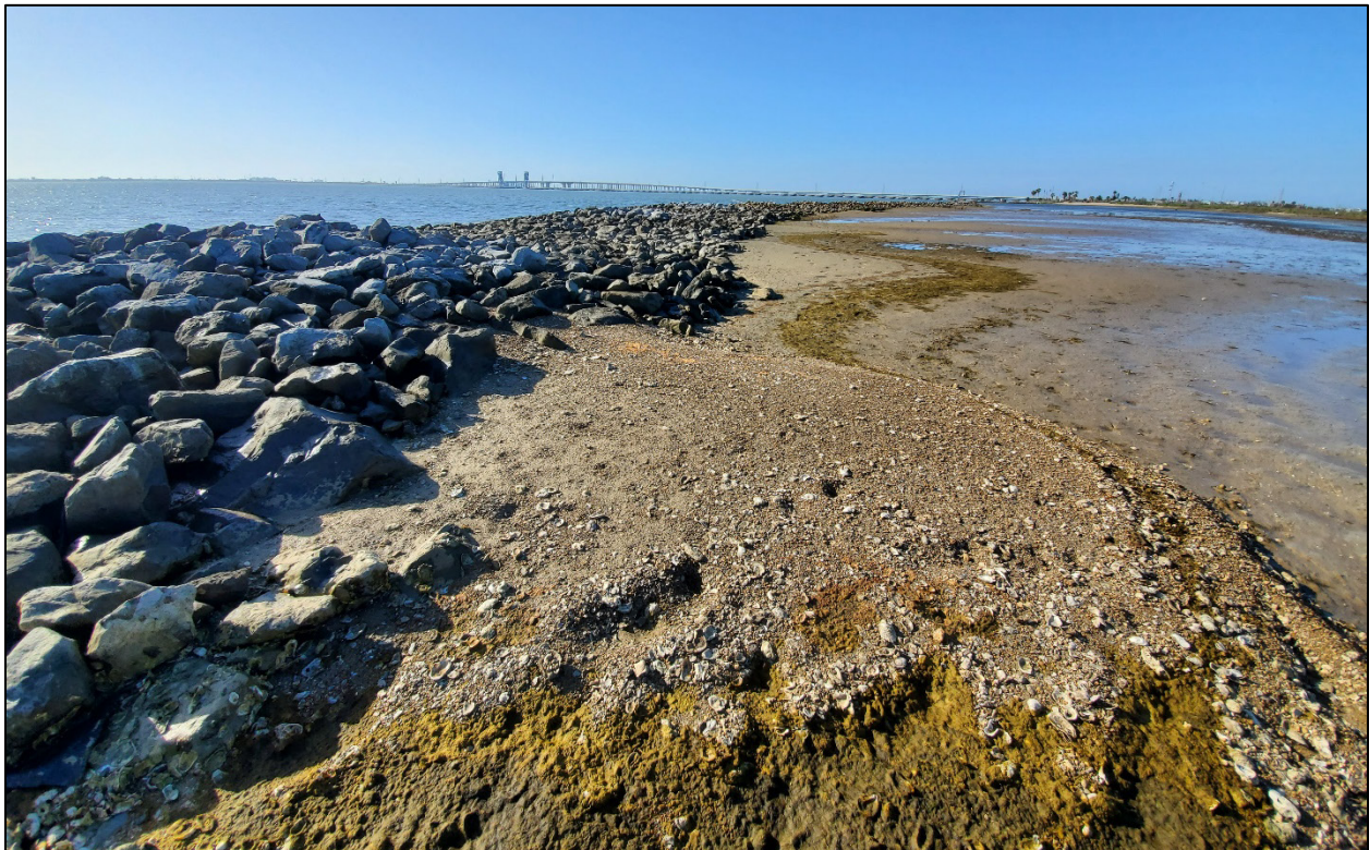
Figure 4. Sediment accretion behind a living shoreline breakwater at Virginia Point in Galveston Bay. Photograph courtesy of Scenic Galveston.
